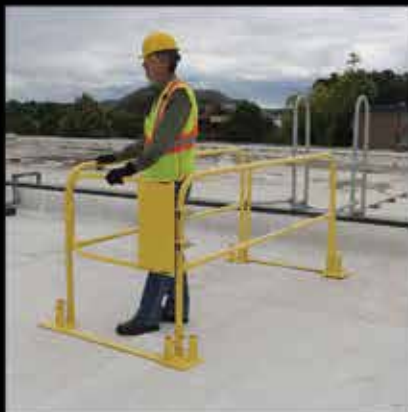
ACCESS LADDER SAFETY
