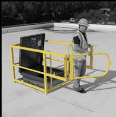
ROOF HATCH SAFETY
